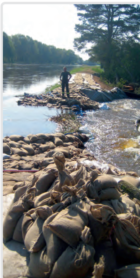
Deichbruch in Arnsnesta
